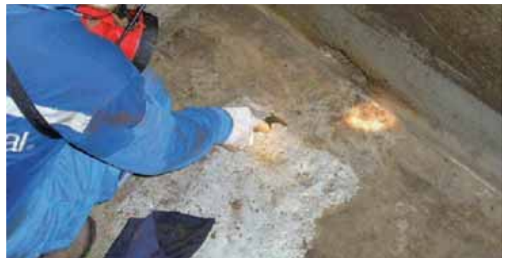
Pitted bottom plate in crude oil tank after 6 years service. Intershield® 300 is still in excellent condition other than dirt and oil stains.
