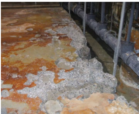
Deteriorated concrete due to chemical attack
