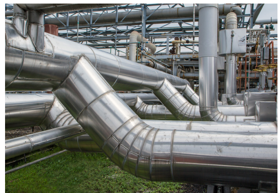
Picture 1: Insulated high temperature piping
